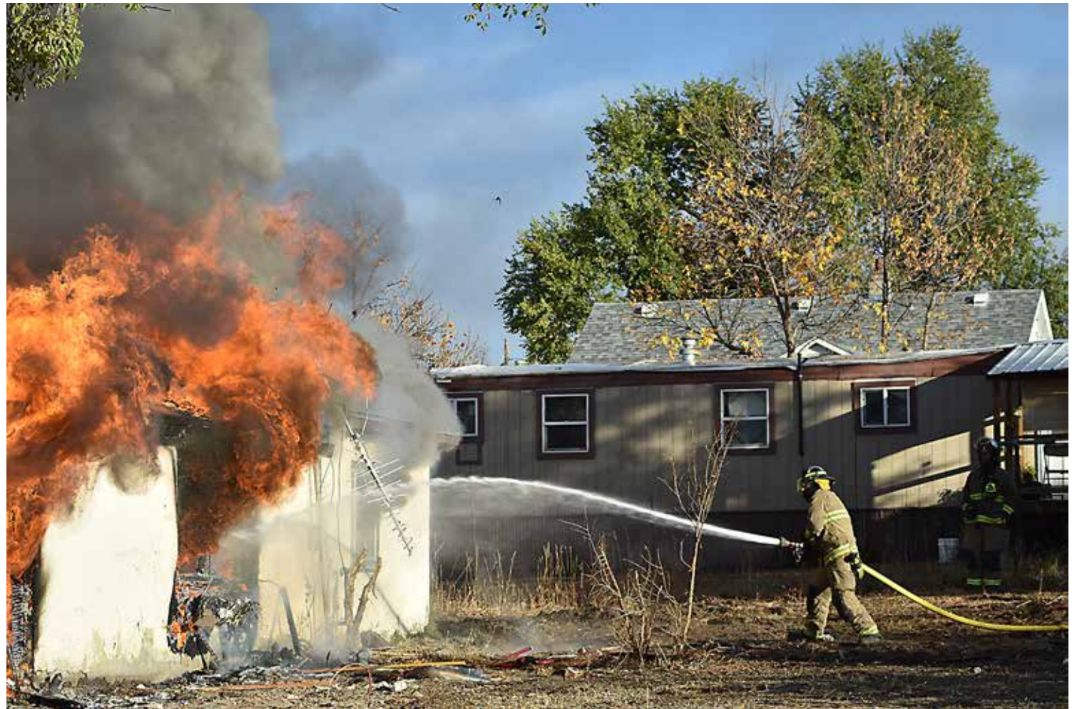
Belle Fourche firefighters got some valuable training when the city partnered with NeighborWorks Dakota Home Resources to remove a dilapidated house on Aurora Street. Photos by Wendy Pitlick of the Black Hills Pioneer.
